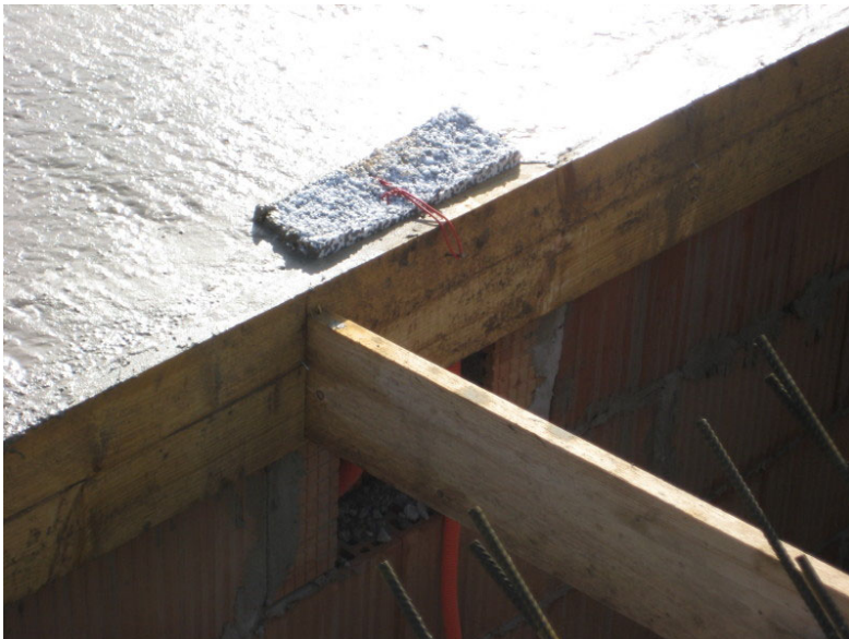
This picture shows a typical styrofoam casting block in-situ. This one is for the installation of heating pipes.
